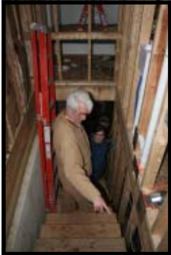
Frank Tilman, instructor at the Career Technical Center, supervises students as they complete electrical work on a new Habitat home on Rogers Street in Cadillac.
