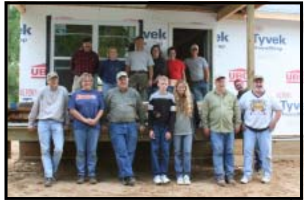
Stacy Proctor (front, third from right) and son Devon relax with volunteers from the DNR after a hard day's work. Soon after this picture was taken, the siding went up. Stacy continues to be an active participant in the building process and is already planning how to use the space in her new rooms. She hopes to be in the home by Christmastime.
