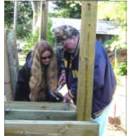
Stacy lends a hand to a DNR volunteer as they build the back porch on her home.
