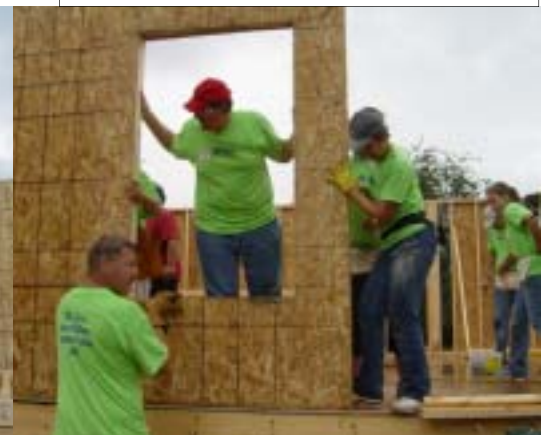
Habitat President Ed Van Alst (left) works with other volunteers to put the wall in place.
