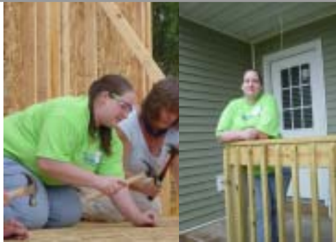
At left, Danielle pounds nails at the Whaley site and at right, looks out from her own new porch.
